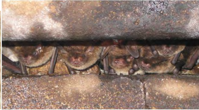
Photo 2: Visible bats within an expansion joint
