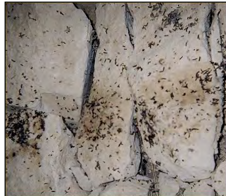
Photo 6: Bat Guano on Riprap
