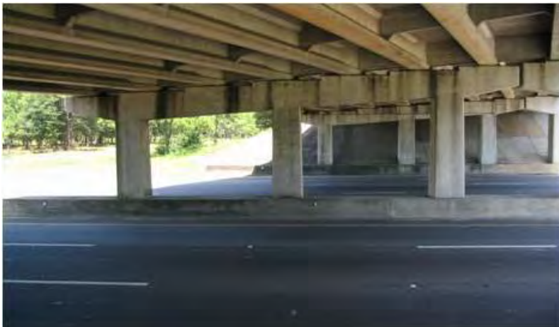
Photo 9: Staining on sides of pier caps
