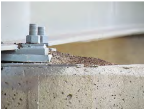
Photo 5: Guano deposit on pier, obscuring structural features.
